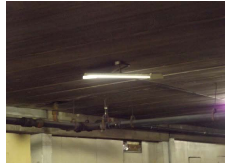
Photo 20 - Typical garage lighting fixture
