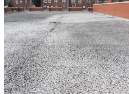
Photo 19 - Membrane over garage
