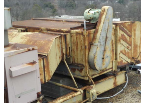
Photo 18 - Corridor HVAC unit
